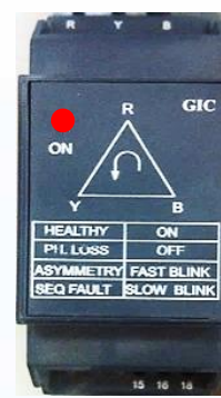
Power Scanner in ODU
